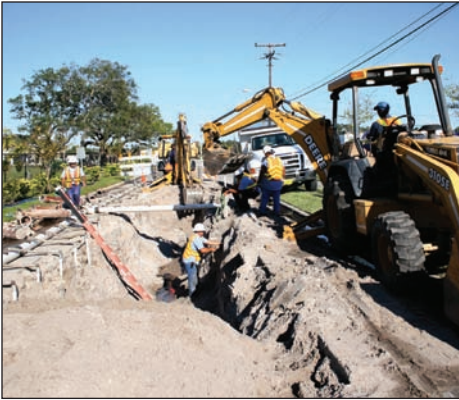
REPLACEMENT of wastewater transmission pipes is undertaken by a City crew in this photo from 2006. Other Melbourne teams continue a program of replacing neighborhood water transmission lines in an ongoing effort to ensure service quality.
