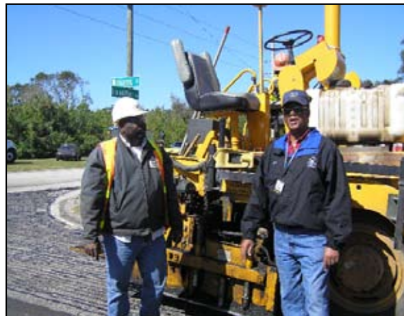
City Construction Inspector Calvin Oliver (r), discusses the recent repaving at Williams Street with APAC Foreman Calvin Pratt.
