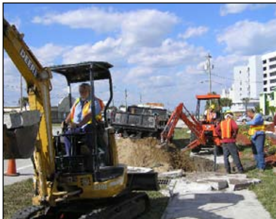
Larry Williams operates the backhoe to dig up the main to cut the valve in. Mueller Services is shown in the background working to install the line stop.
