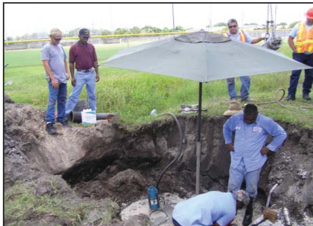
Water Distribution Foreman Tim Hedrick (left) and Wastewater Collection Foreman Perry McThenney observe as Robert "Colgate" Coger and Odell Wadlington work to connect the smaller reuse main to a larger one. Rubin Rosada and Charlie Packard prepare to insert the tapping device.
