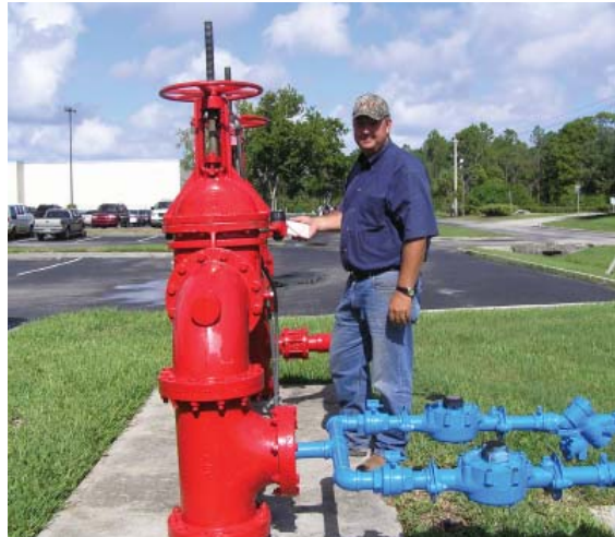
Environmental Compliance Technician Tim Mulligan checks the testing tag of the backflow prevention devices at the Harris facility on Wickham Road.
