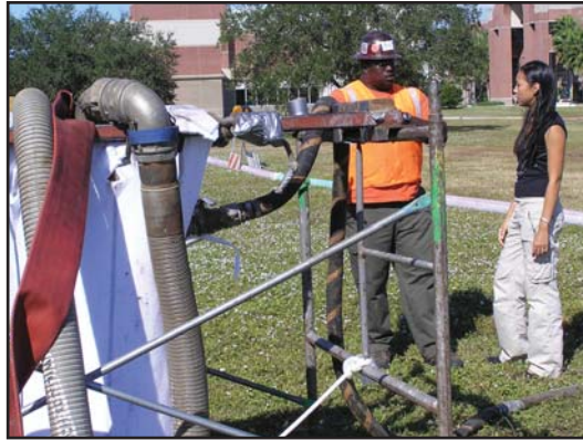
Insituform Foreman James Cringley provides an update to City Utilities Engineer Michelle Shoultz.
