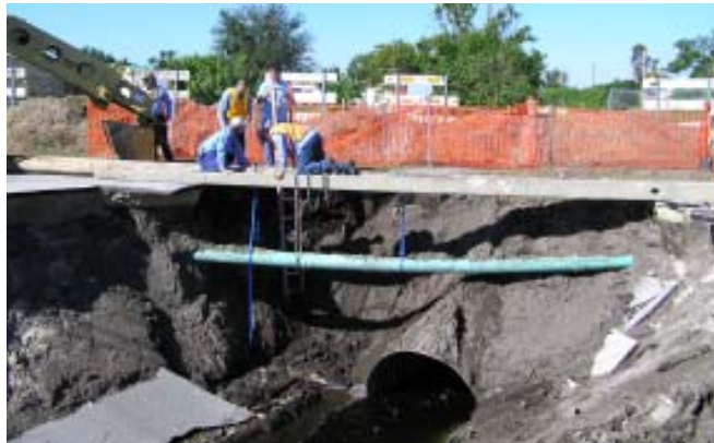
At the south end of Croton Road, crews from Wastewater Collections and Streets & Stormwater attach sewer pipe to a pole. Gator Hembree and Matt Simon are on top of pole, while Larry Blumenburg, Butch Burke and Josh Baker assist.
