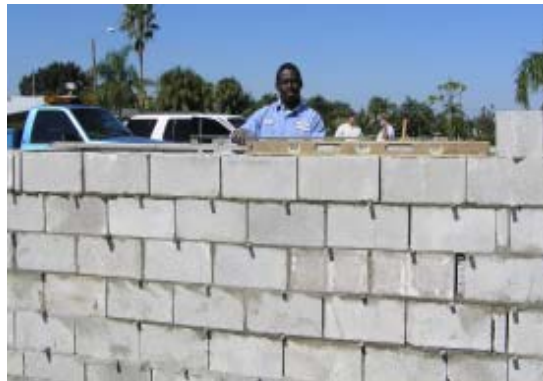
Manny Parker of the Streets and Stormwater Division works on new dumpster enclosure at Florida Tech. The previous enclosure was demolished during the wastewater line repairs.
