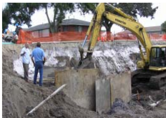
Superintendent Tom Hogeland (l) discusses the sewer line replacement project with Bruce Robinson, foreman for Derrico Construction.
