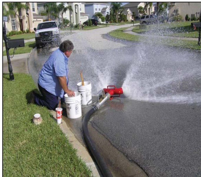
John Hummel adds chemical to dechlorinate the water being flushed in one of the recent pilot test areas.
