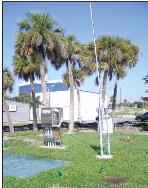
The existing lift station at Front Street Park is readied for dismantling as construction begins on the new station that will replace it.
