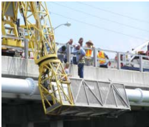
Tim Hedrick, seated on the pipe, and Robert Sigman prepare to make repairs. Other division staff observe and assist.
