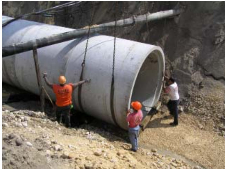
Workers with RKT Constructors work on placing one of the sections of new stormwater pipe under Laurie Street.
