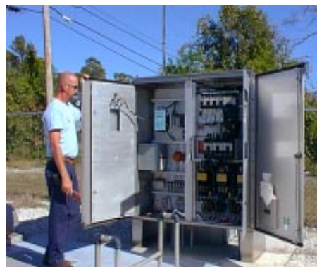
Above, electrician Mike Brink checks the control panel at Lift Station #23.
