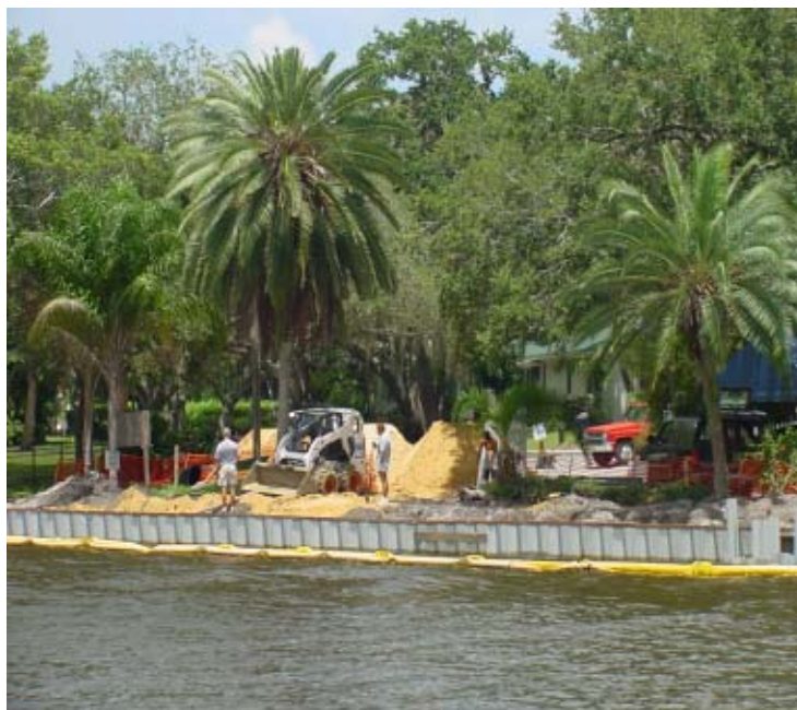
Work proceeds on the new seawall at the end of Houston Street.
