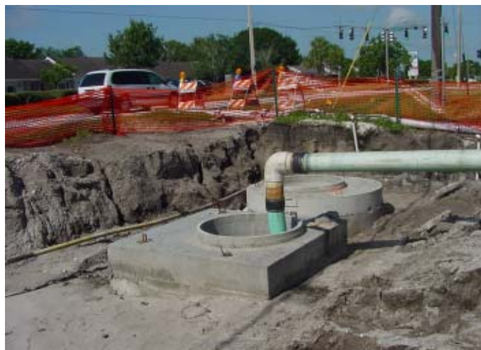
The well-point dewatering system temporarily discharges groundwater into the new storm drainage structure at Bell Avenue.
