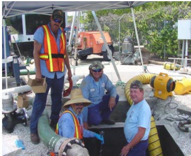
Crew working inside the wet well includes, from left, Jim Symonetta, Butch Burke, Kevin Pugh and Charlie Charles.
