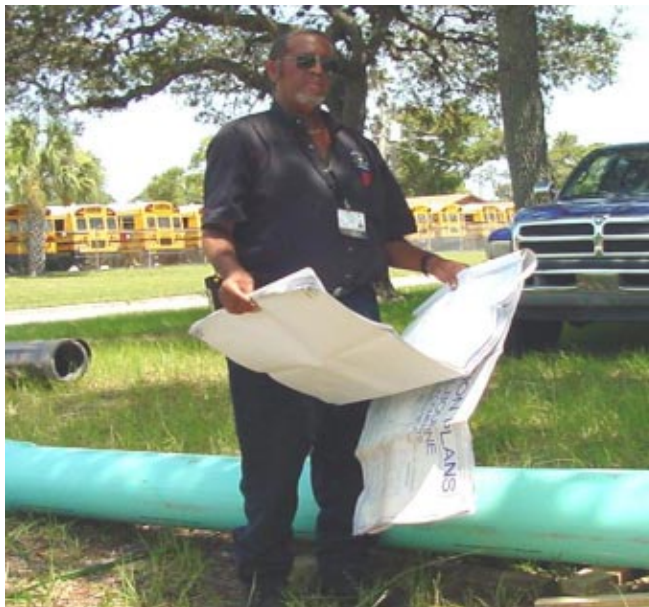
City Engineering Inspector Calvin Oliver reviews plans for the project as a section of PVC pipe ready for installation rests on the ground behind him.
