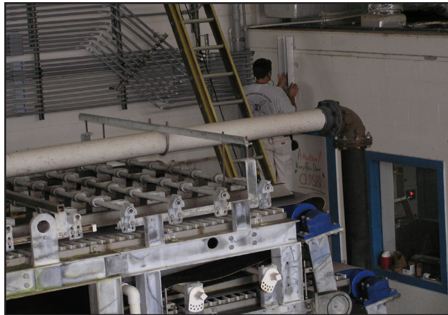
Worker with FIE installs conduit in belt press room at the D.B. Lee Water Reclamation Facility.
