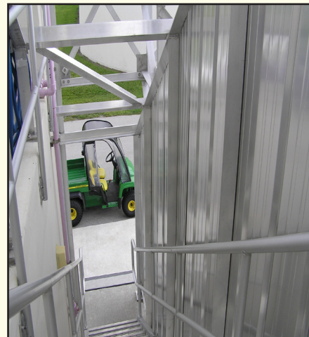
Looking down the influent structure stairwell, the new aluminum shield will protect operators entering and exiting the second-floor control room during strong storm events.
