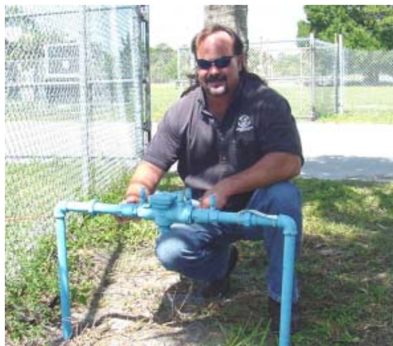
Environmental Compliance Technician Darrell Manchester checks backflow prevention device.
