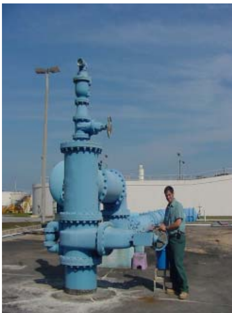
Hector Nazario, operations supervisor at the Grant Street plant stands next the injection well that will be undergoing mechanical integrity testing.
