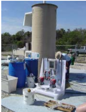
The on-site delivery system is set up for testing.
