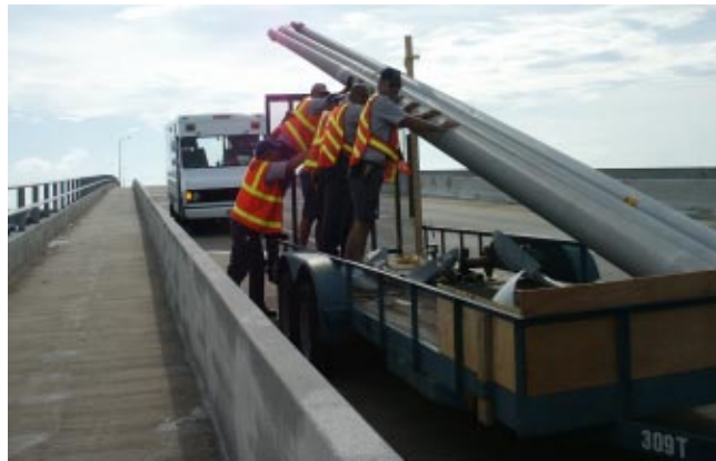
Facilities Maintenance crew collects 45-foot long, 400-pound street light poles, 11 of which fell down on the Melbourne Causeway following Hurricane Frances. The crew includes Greg Valenti, Don DeLoach, Lasalle Randall, John Striepe, George Wood, Gene Henderson and Superintendent Marv Sharp.
