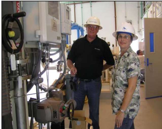
George Varall (left), of Hazen & Sawyer, and Martha Campbell inspect one of the ozone generators.
