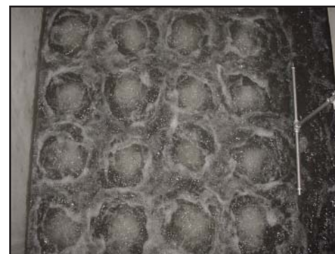
A bubble test is performed in the contactor to verify the diffusers are operating correctly.
